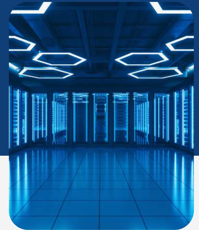
5. Data Centre Equipment
